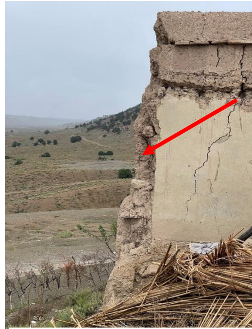
Figure 2-14. Failed section of Pakhsa wall
