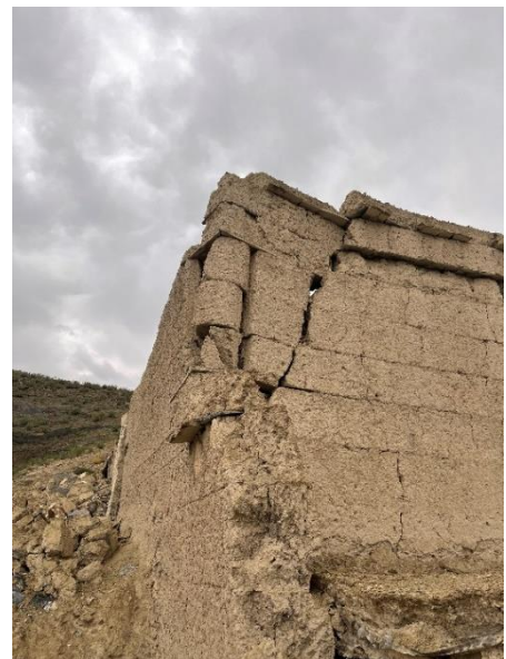
Figure 2-10 Example 2 of corner detachment
