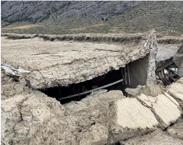
Figure 2-13. Failed section of multilayered roof.
